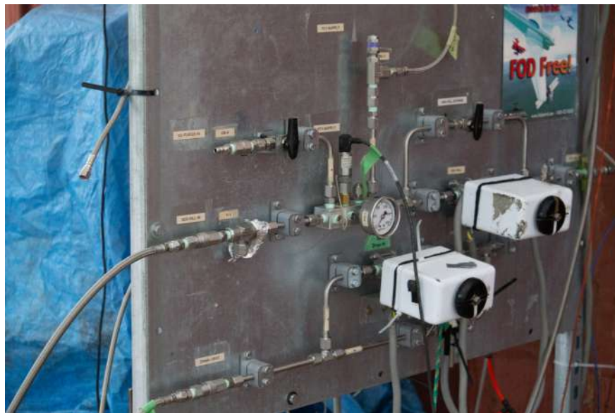
Figure 11.12: Assembled nitrous oxide fill panel
